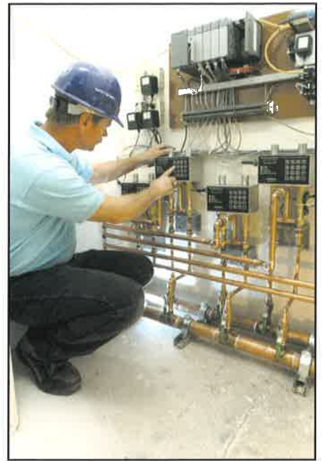
The mechanical closet features six valves that deliver water equally to each showerhead zone.
